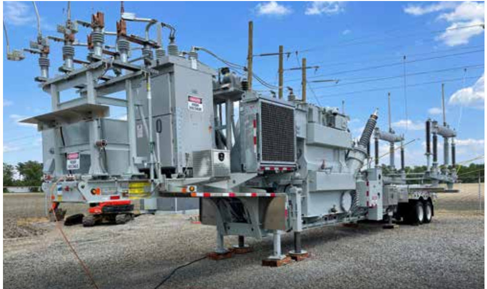
Should a substation fail, the mobile unit can be moved into place within hours.
